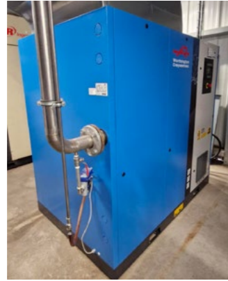
New compressor at Mortagne site
