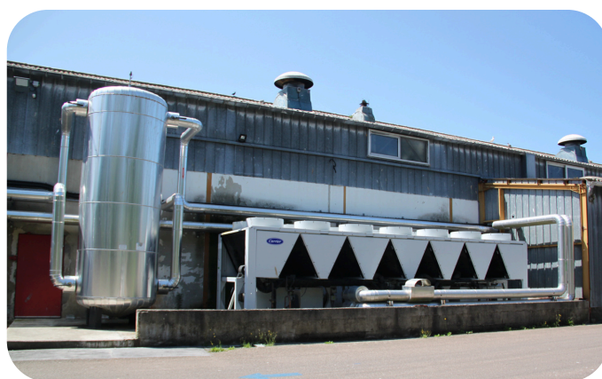
Heat recovery system
