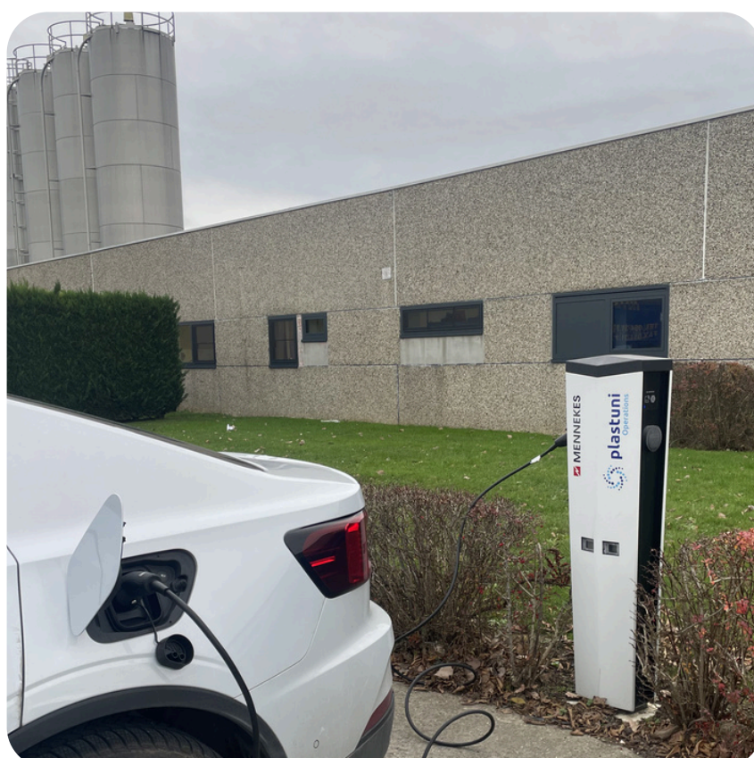
Electric vehicle charging stations - Plastuni Operations
