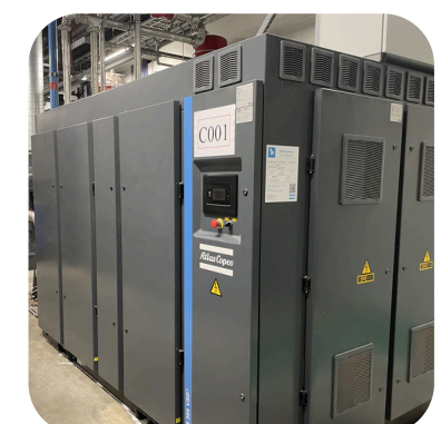
New compressor - ANL Wellen
